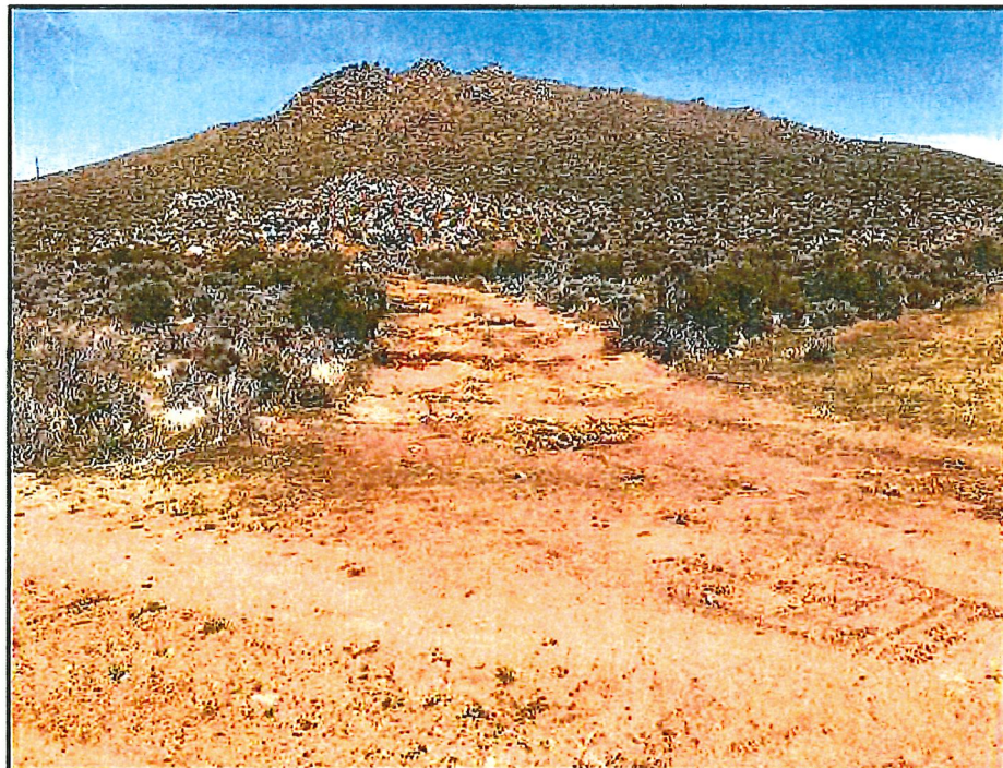
Portion of new access that branches off of existing sewer line road where vegetation was crushed, but earth was not "regraded."
